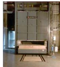
Car Bottom Furnace
