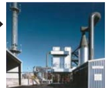
Air Pollution Control System
